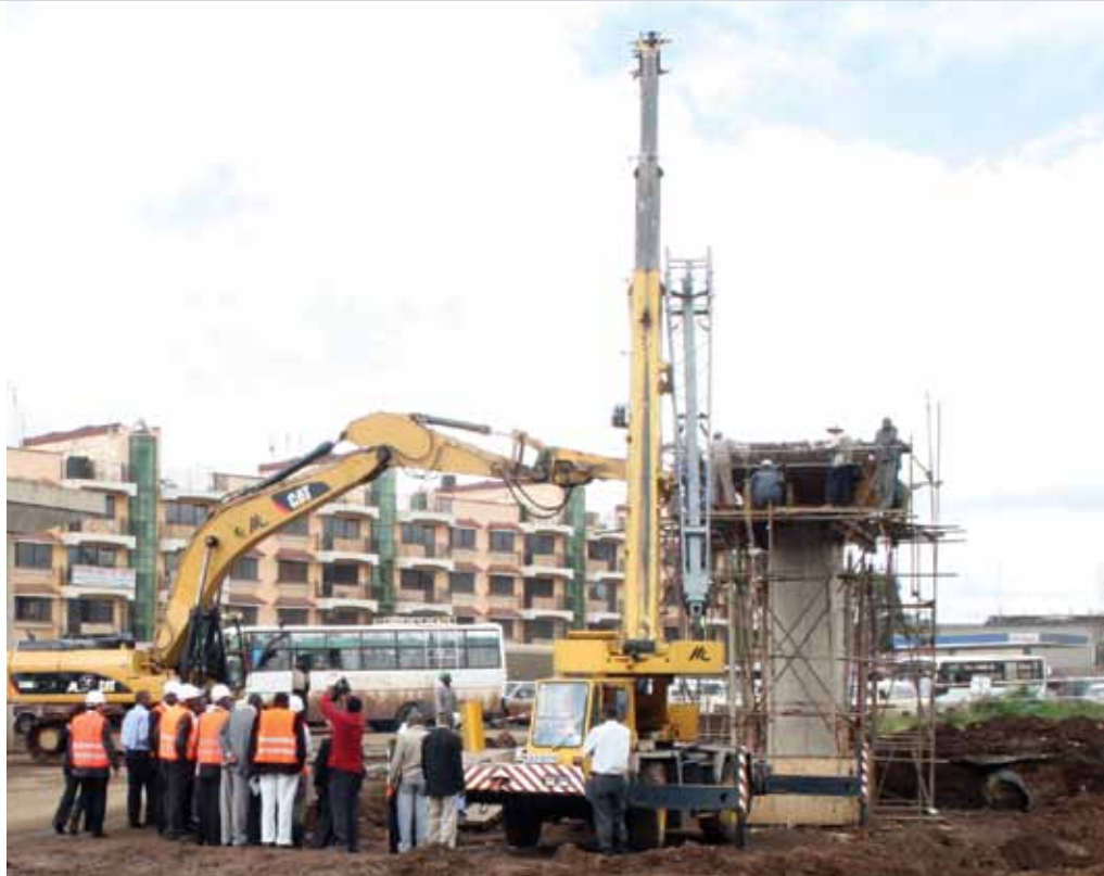
A CAT truck busy at a road construction site. Most of its functions rely on hydraulics.
